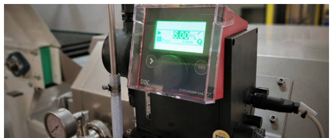
Automatic chemical dosing pumps
